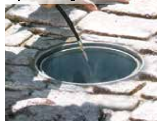
Pipe cleaning hose
