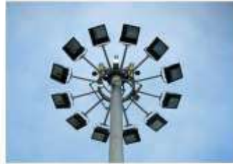
Solar Street Light- High Mast
